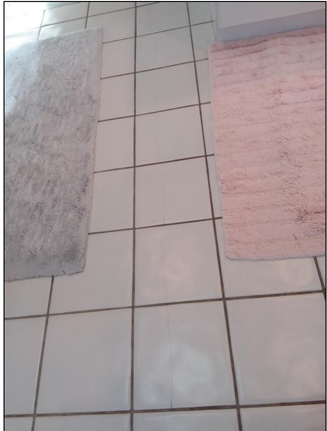
Cracked floor tiles
