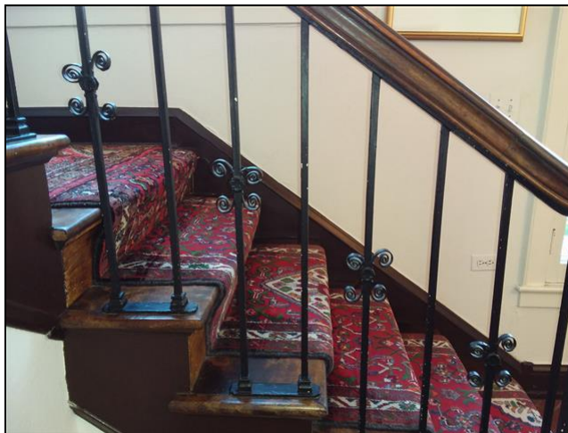
Wide spacing at stair railing
