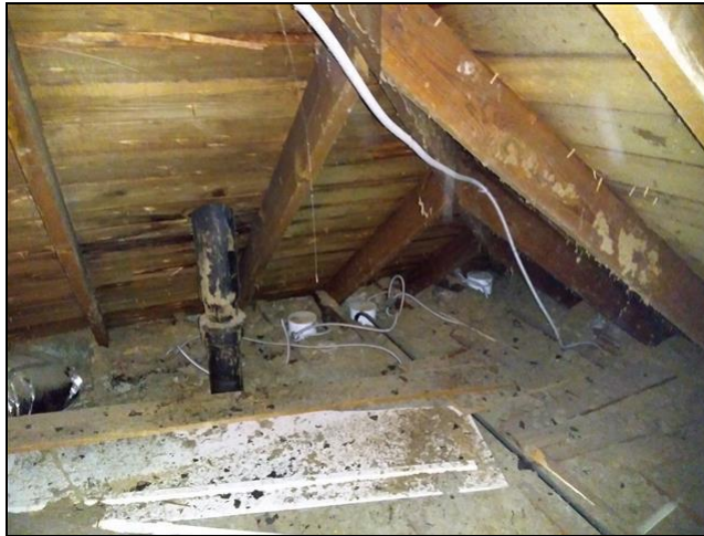
Amateur attic wiring
