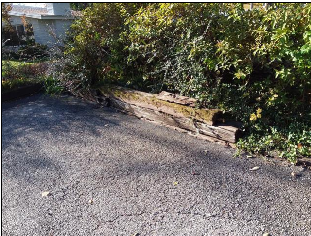
Failing retaining wall
