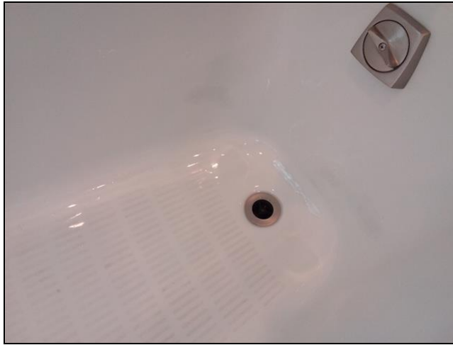
Missing tub drain stopper
