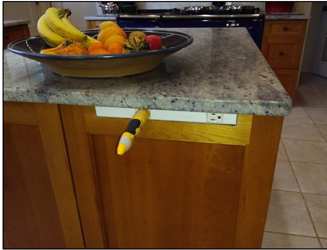
No power at outlets
