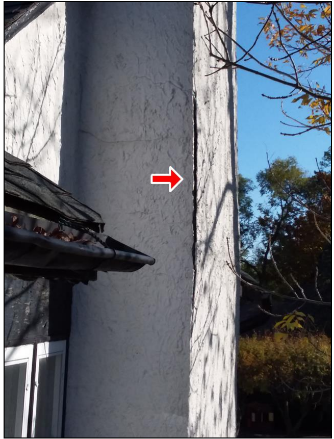
Cracked stucco at chimney
