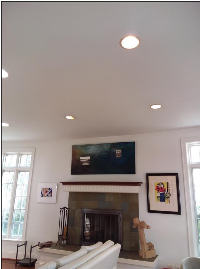
No smoke detector in family room
