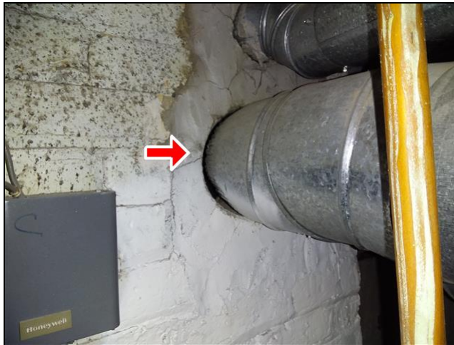
Large gaps at chimney connection
