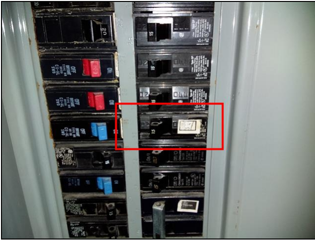
Non-GFCI breaker for tub motor
