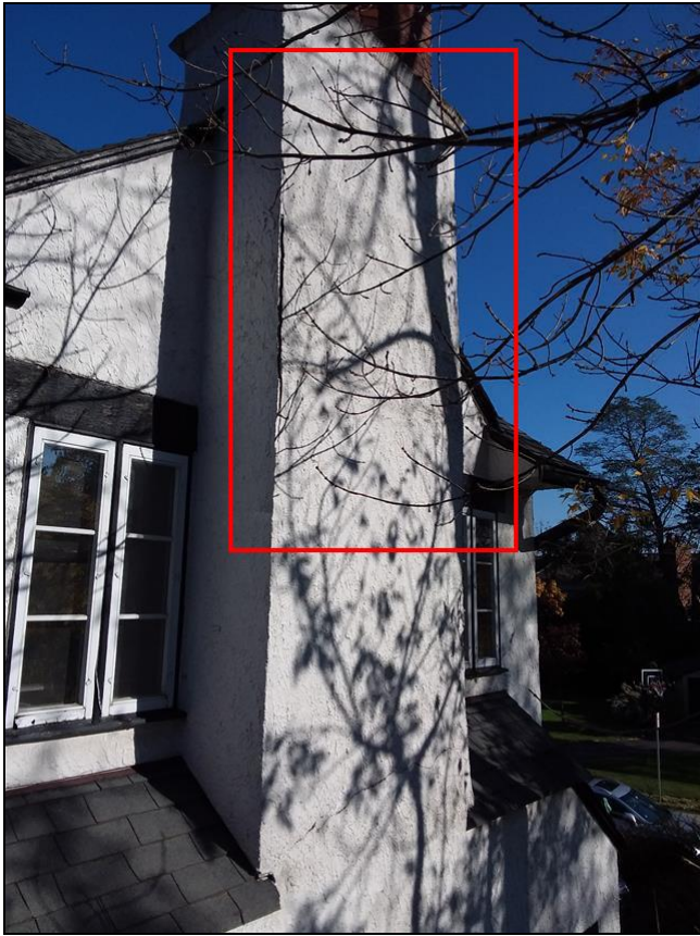
Deteriorated stucco at chimney
