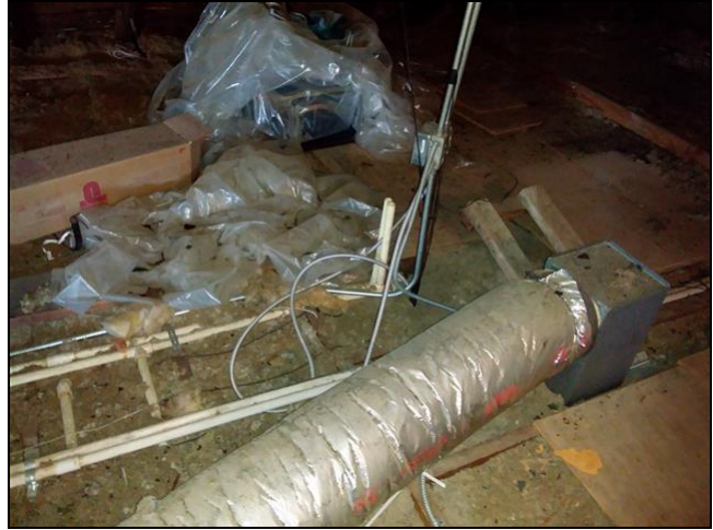
Amateur attic wiring
