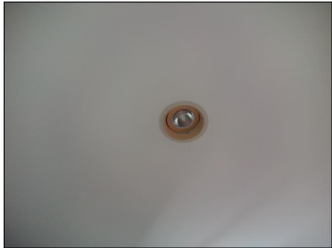
Family room ceiling light out
