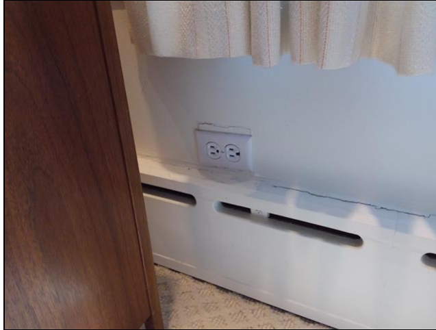
Outlet installed over radiator
