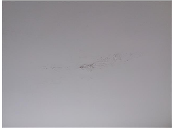
Moisture damage at ceiling
