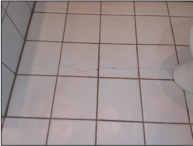
Cracked floor tiles
