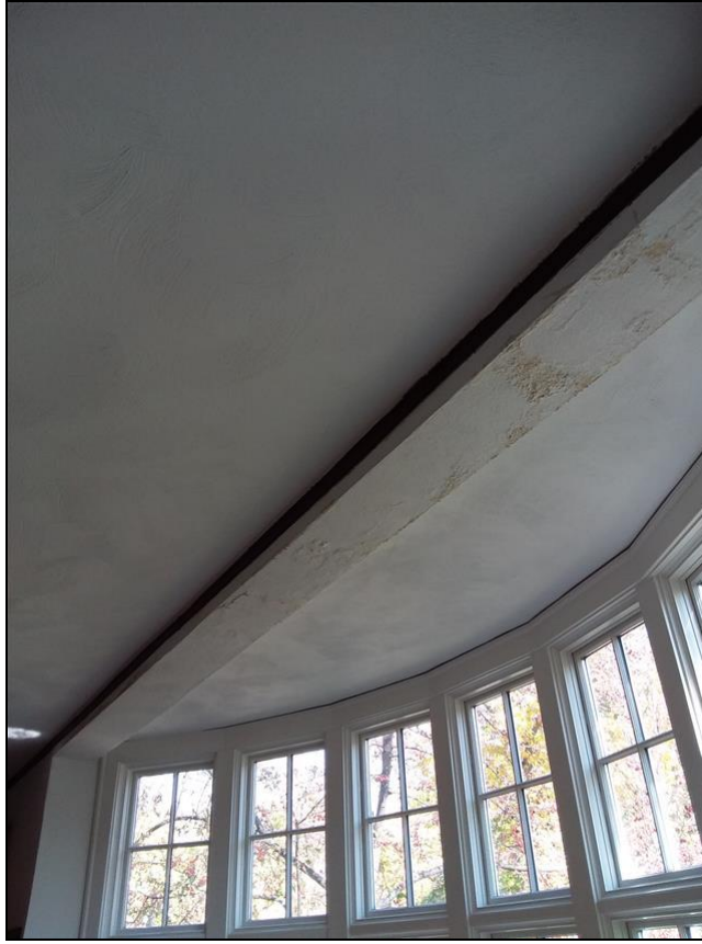
Water damage at ceiling
