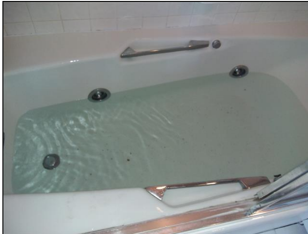
Debris in tub jets
