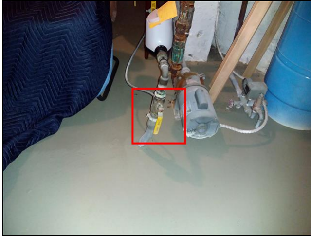
Main water shut-off
