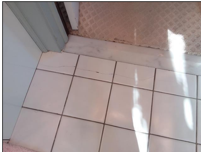
Cracked floor tiles
