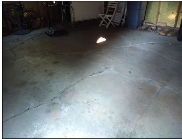
Cracked garage floor
