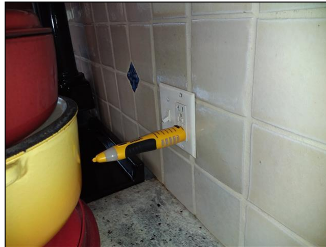
No power at outlet
