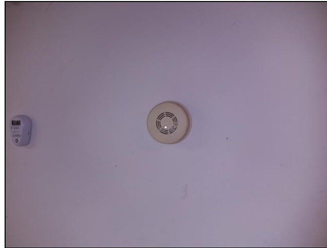
Old, yellowed basement smoke detector
