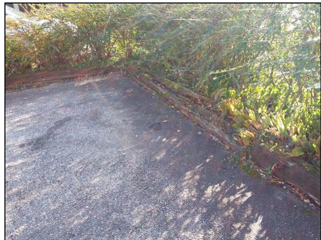
Failing retaining wall
