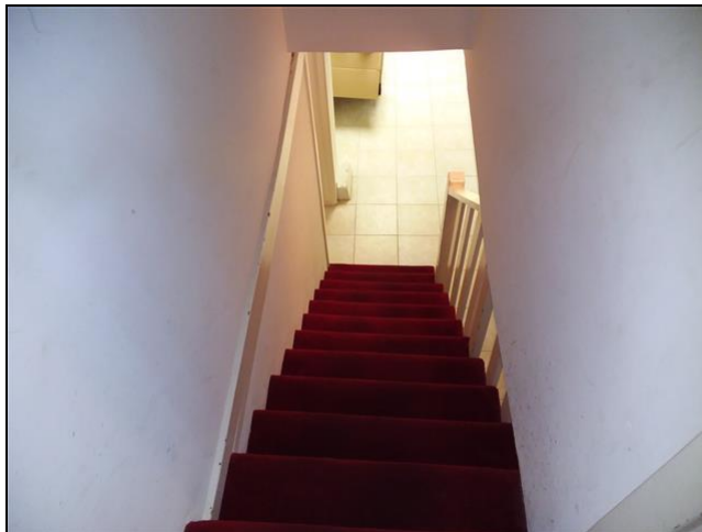
Add full railing at basement stairs
