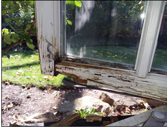
Rotted wood window
