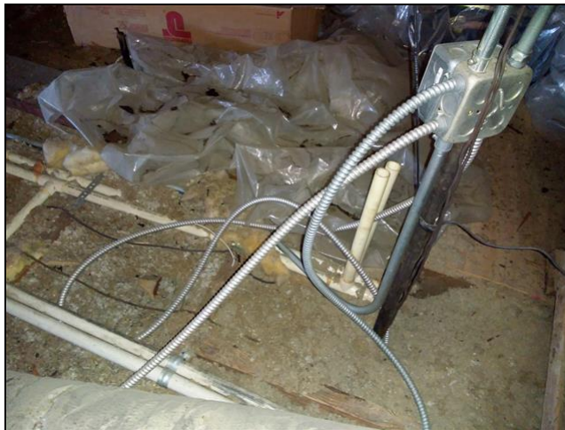
BX wiring in attic
