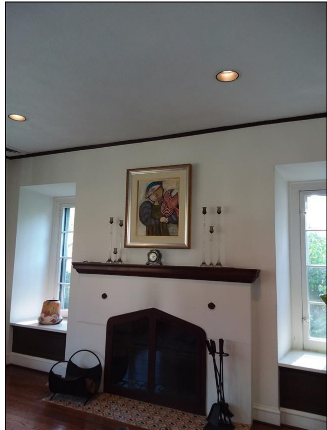
No smoke detector in living room
