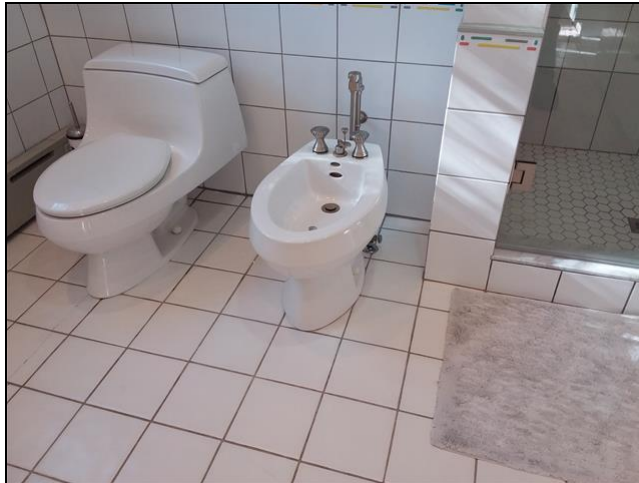
Bidet loose on floor
