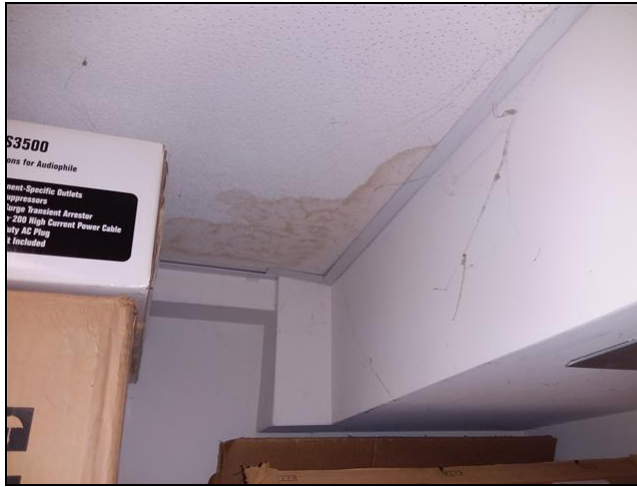
Water stains at ceiling tile
