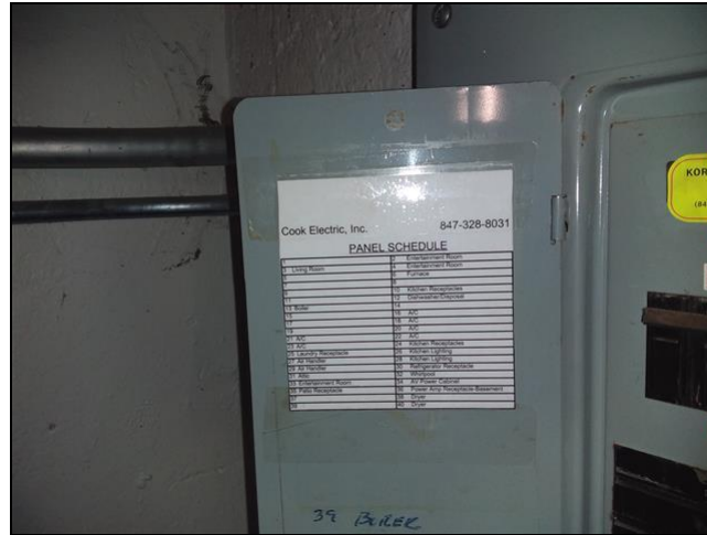
Incomplete circuit directory at panel
