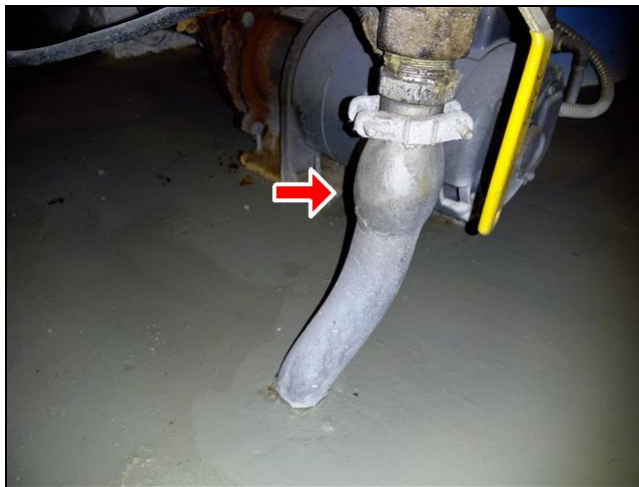
Lead water service piping
