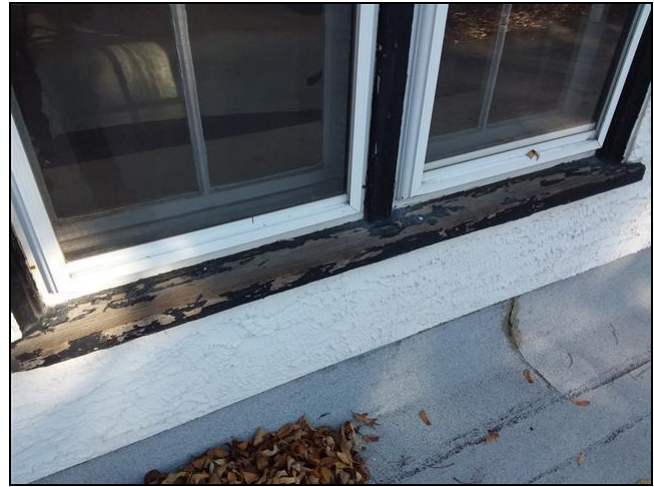
Deteriorated trim paint
