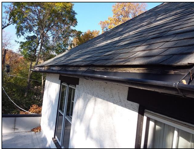
Exposed wood at fascia
