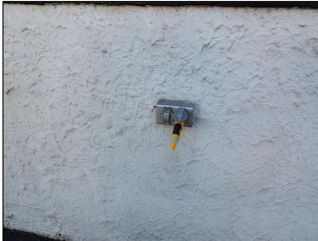
Non-GFCI exterior outlet
