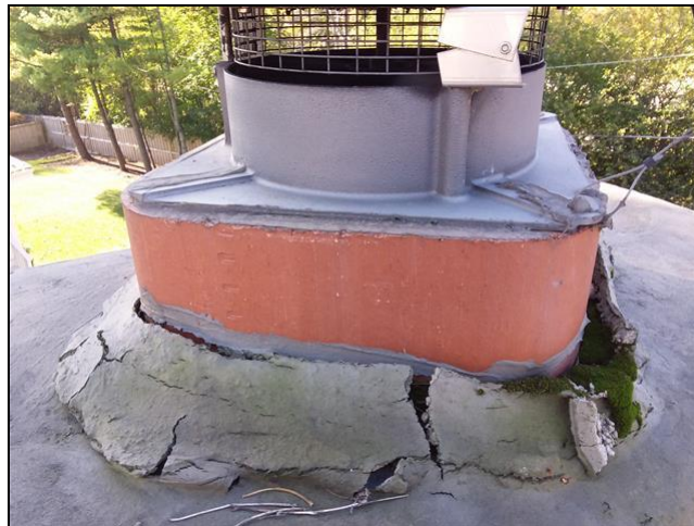
Cracked, deteriorated mortar wash
