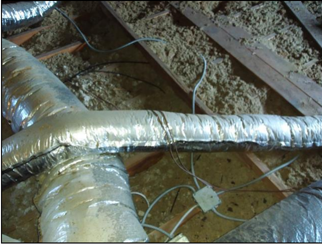
Amateur attic wiring
