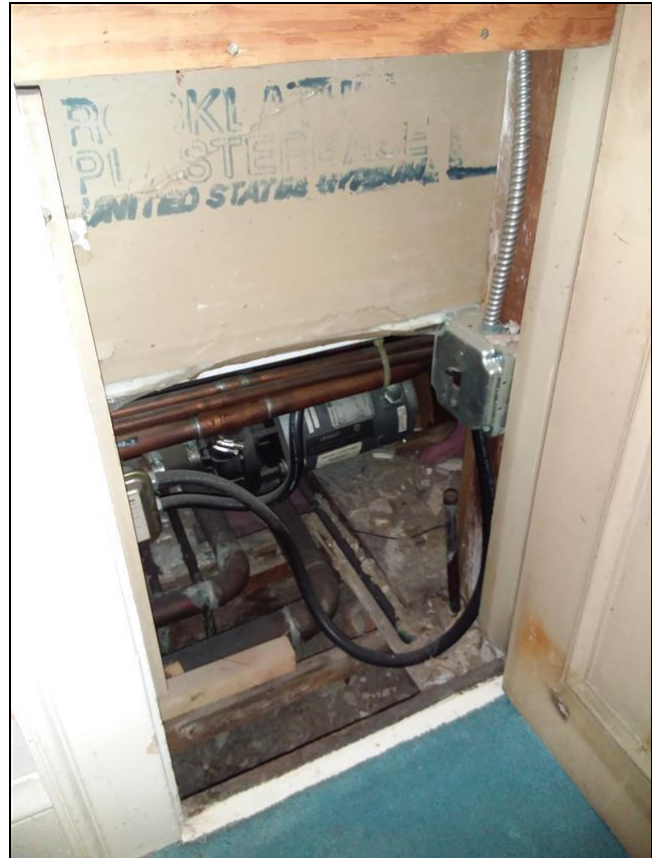
No GFCI protection at tub motor
