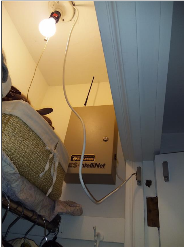
Improperly installed electrical wiring
