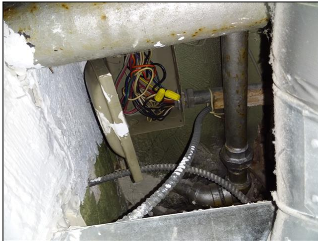
Open junction box
