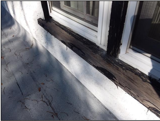
Deteriorated trim paint
