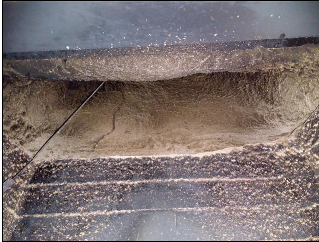
Dirty family room fireplace flue
