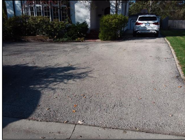
Worn, deteriorated asphalt driveway
