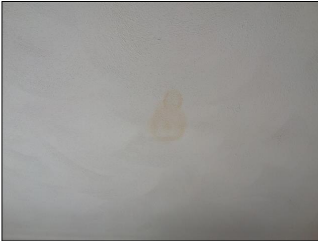
Water stain at ceiling
