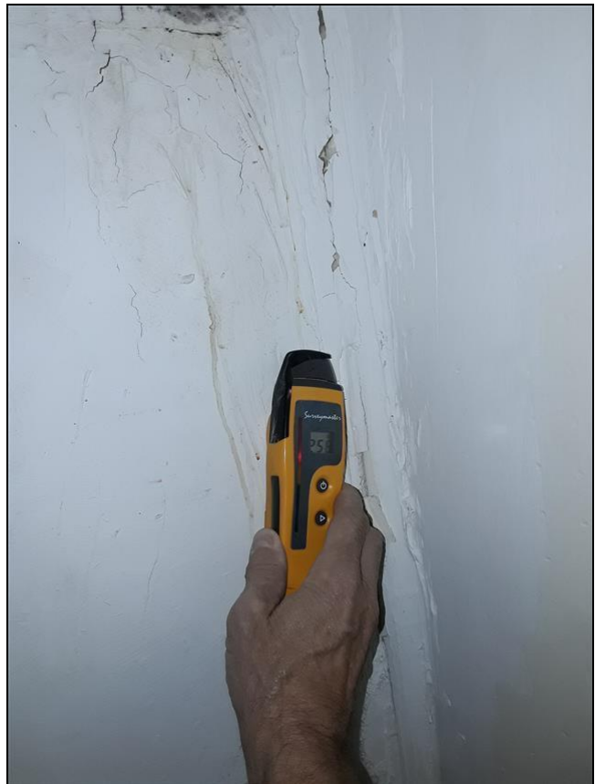
Elevated moisture levels confirmed
