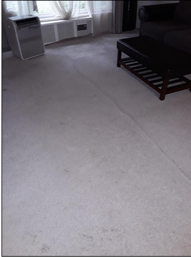
Old, loose and torn carpet
