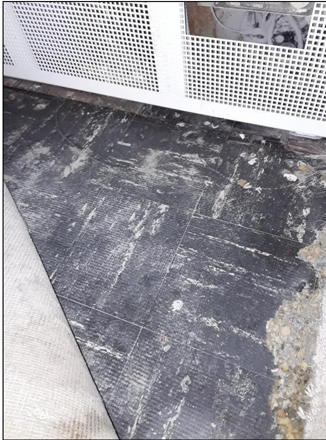
Asbestos floor tiles
