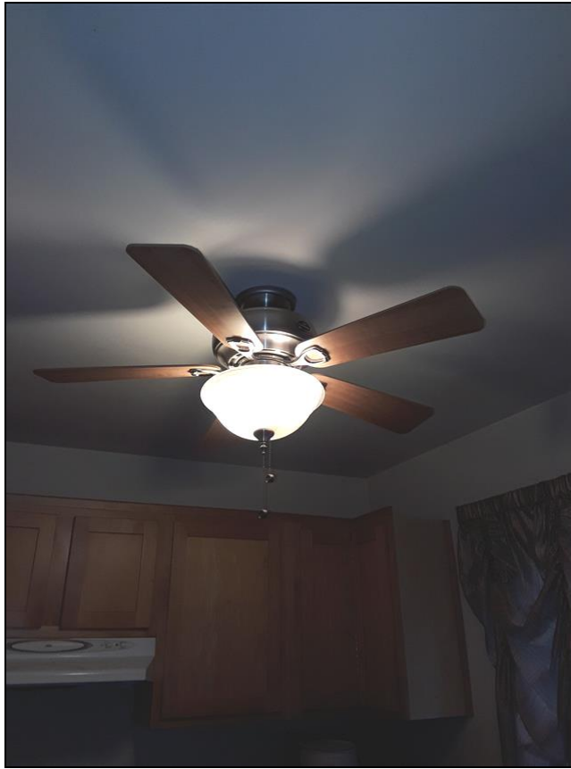
Ceiling fan not working
