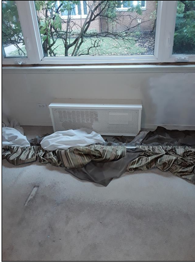
Fan not working
