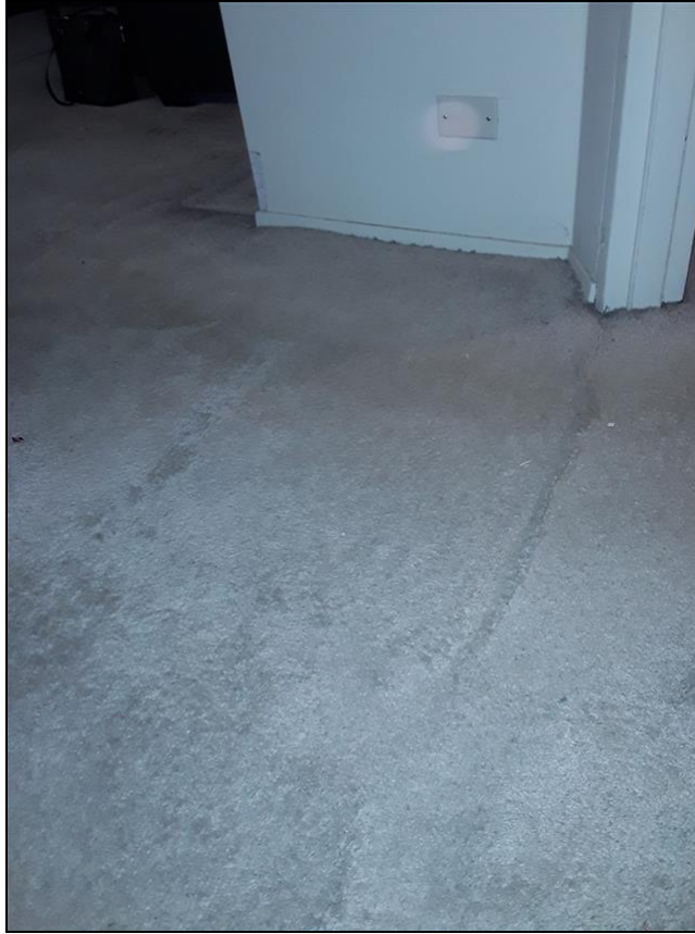
Loose or damaged wood sub-floor
