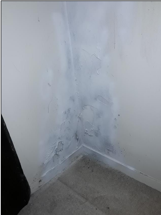
Water damage at living room wall
