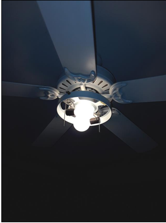
Missing light globe
