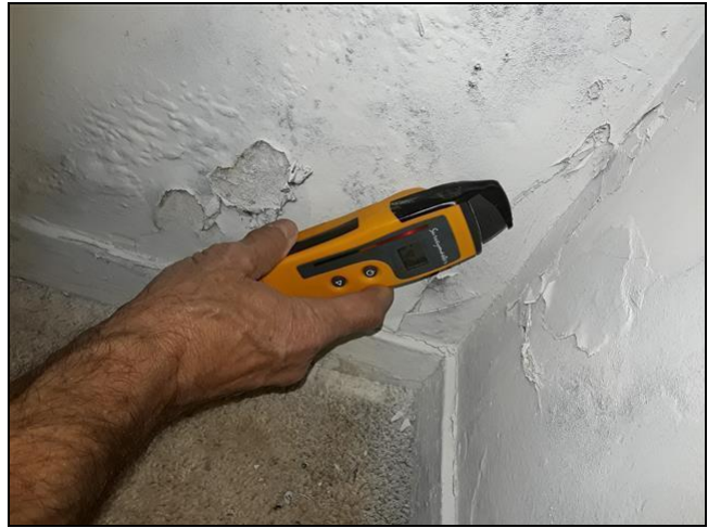
Elevated moisture levels confirmed
