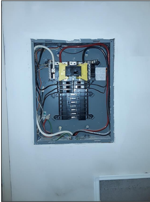
Main electrical panel with cover removed
