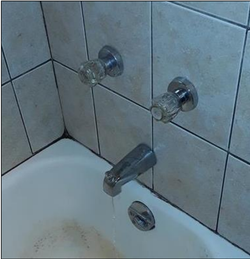
Water drips continuously
