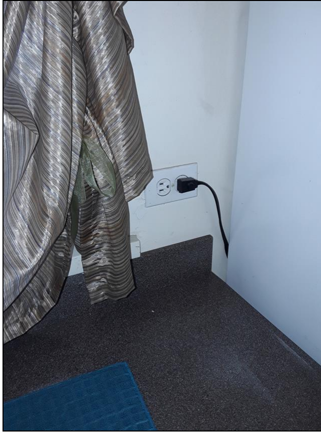
Non-GFCI kitchen counter outlet
