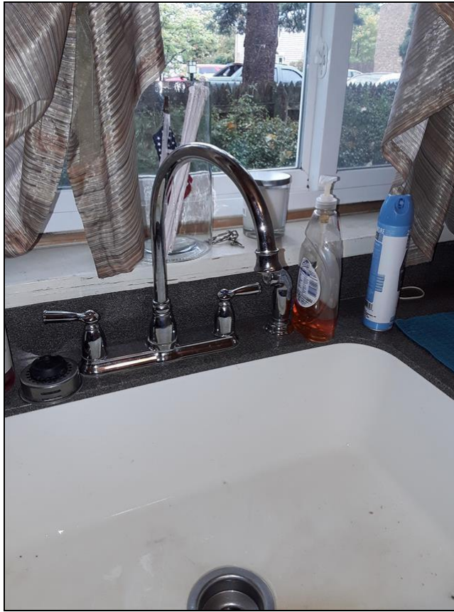
Faucet drips continuously
