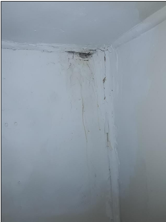
Water damage at closet
